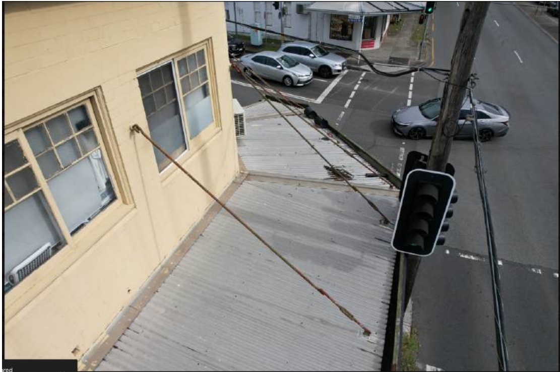
Fig.3 Awning from a drone. Rust seen in Tie rods
