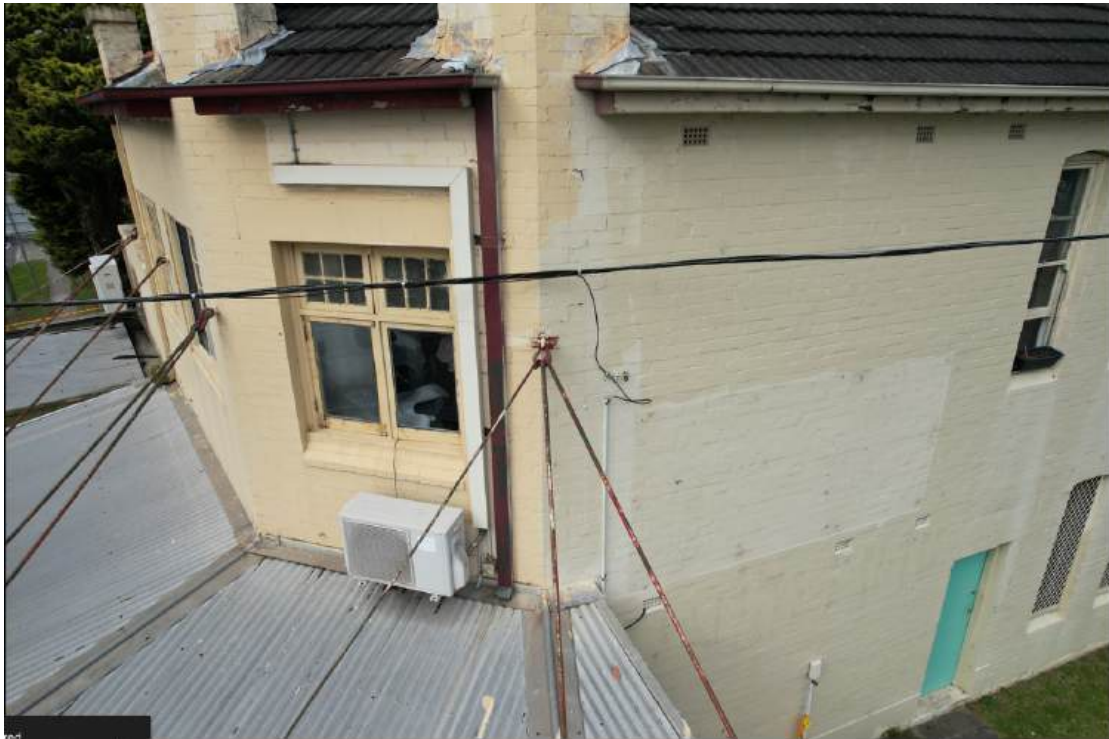
Fig.1 Awning from a drone. Shows some damage to the wall where the awning is braced.
